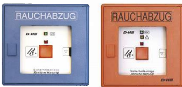
Fig. 4: Manual call points (orange and blue) for smoke extraction and manual control
